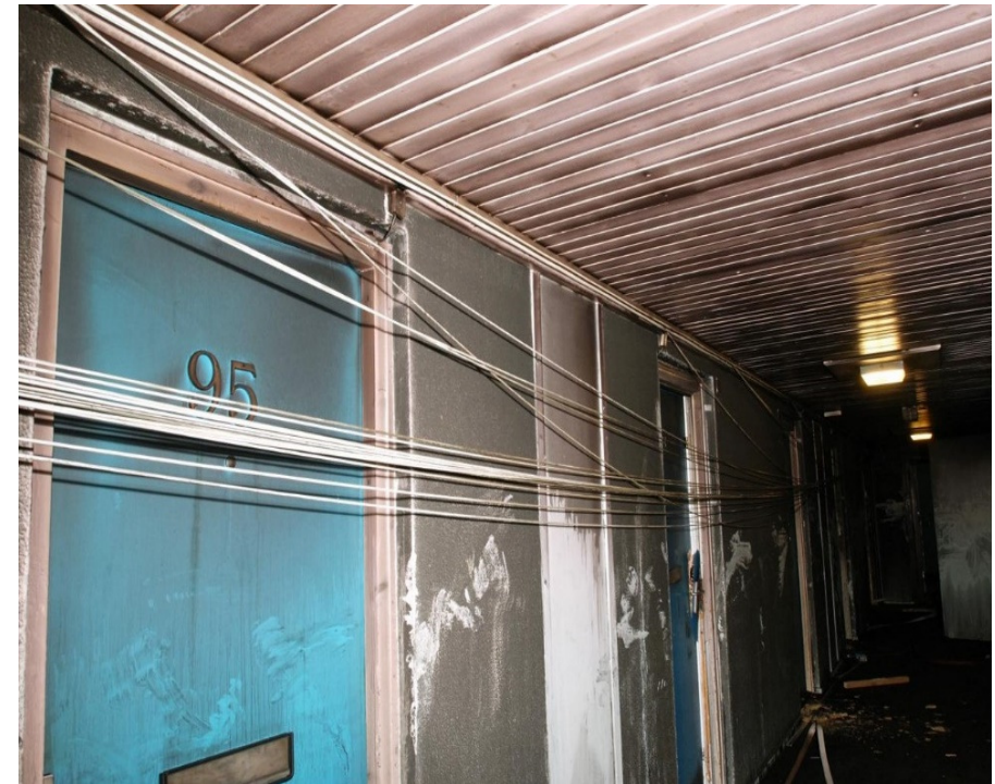
Shirley Towers – Southampton 2010. Two firefighters killed due to cable entanglement.
