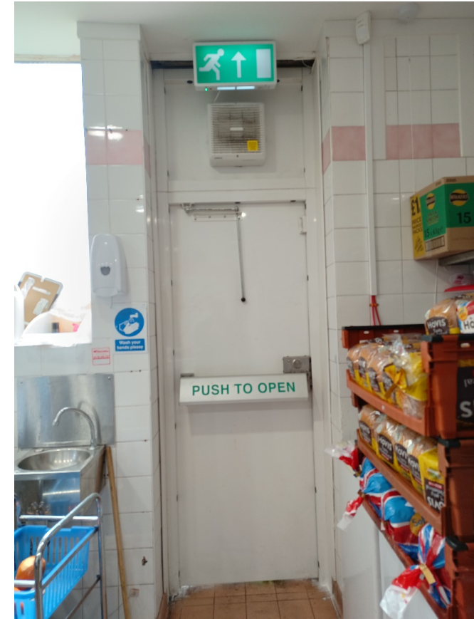
Improved Compliance with Security Assessment and Fire Assessment
